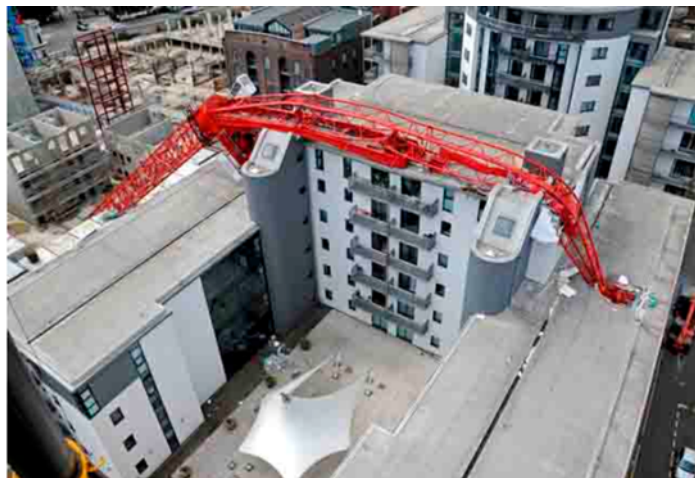
Figure 1 The toppled tower crane lays across residential apartments
