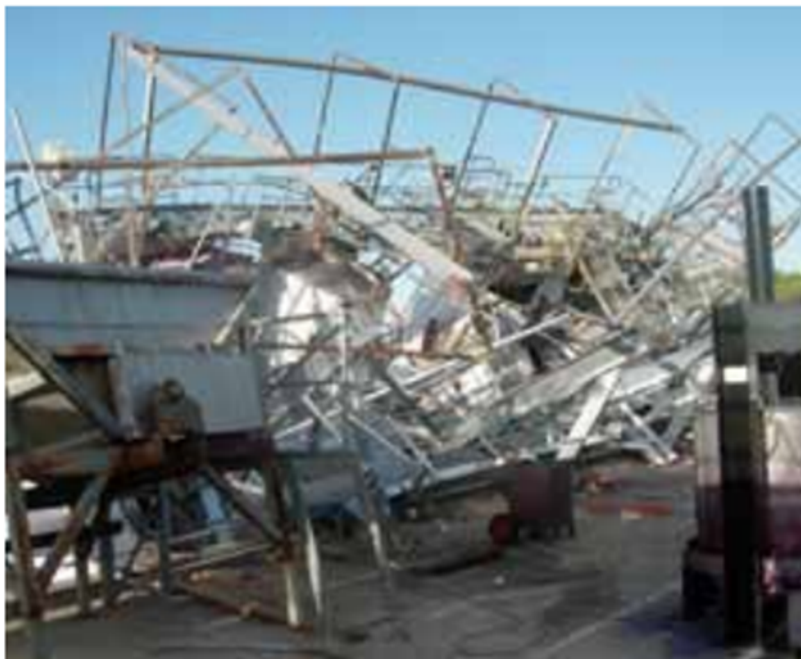
Figure 1 Wirra Wirra Production Facility Post-Incident
